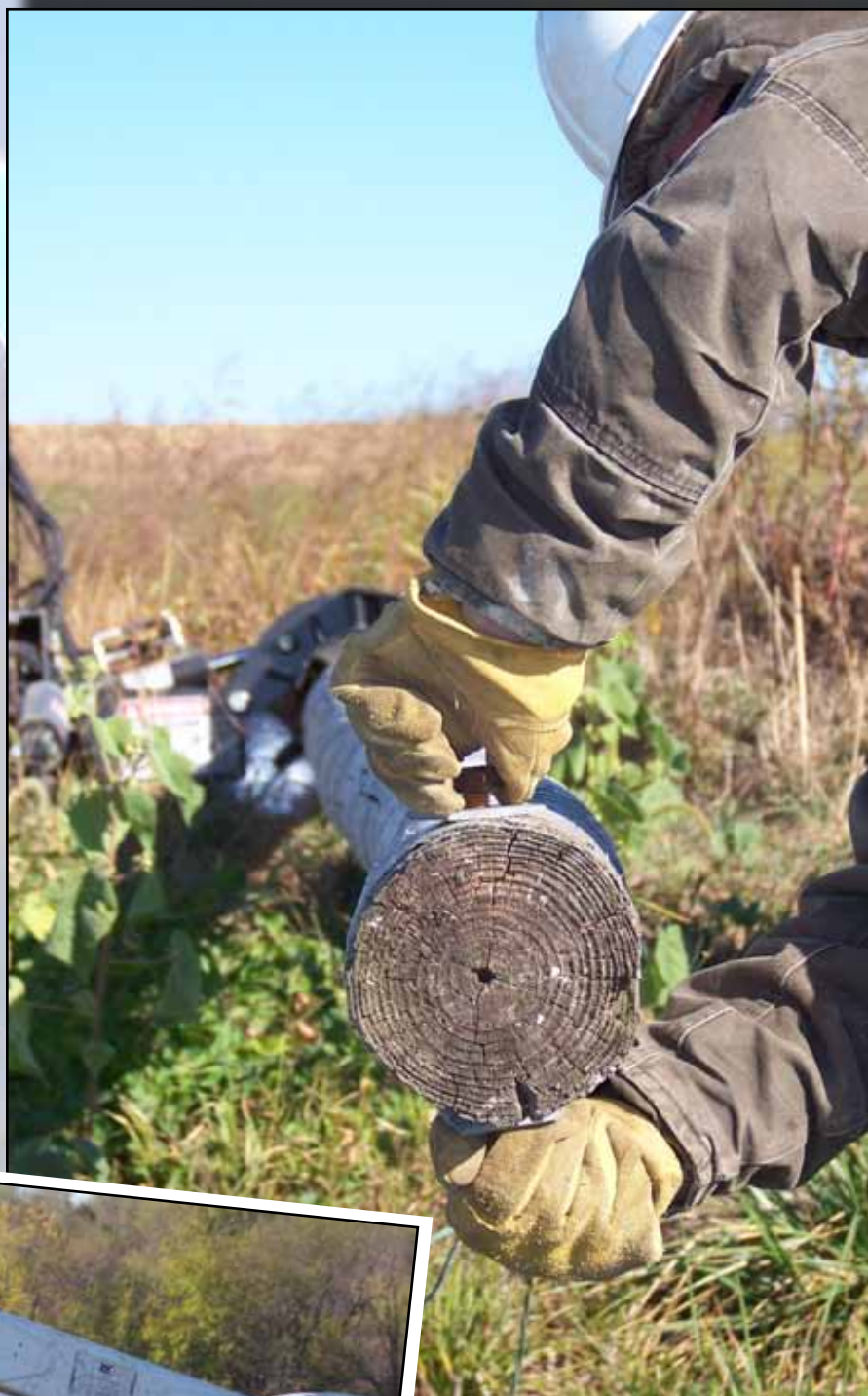
OUT WITH THE OLD... WCE crews work to retire one of the many unused services within the cooperative's service area. (Top left photo) Journeyman Lineman Tim Frerking cuts a guy wire attached to a pole in preparation of removing a service line. (Bottom photo) Eric Wegener works an unused pole out of the ground. (Top right photo) Derek Cole removes hardware from a felled pole.
